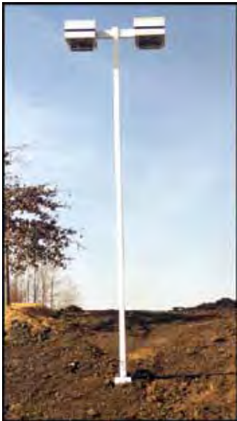
Installed Light Standard Figure 10-2
