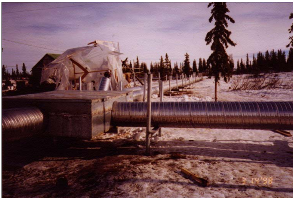
Figure 4.5 Arctic Pipe with Helical Piers as a Foundation in Noorvik, Alaska (ANTHC, DEHE)
