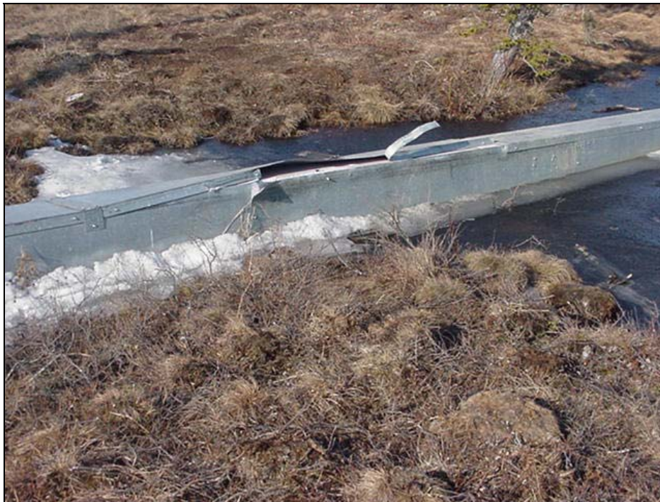
Figure 4.2 Damaged Utilidor on Grade, Noorvik, Alaska (ANTHC, DEHE)
