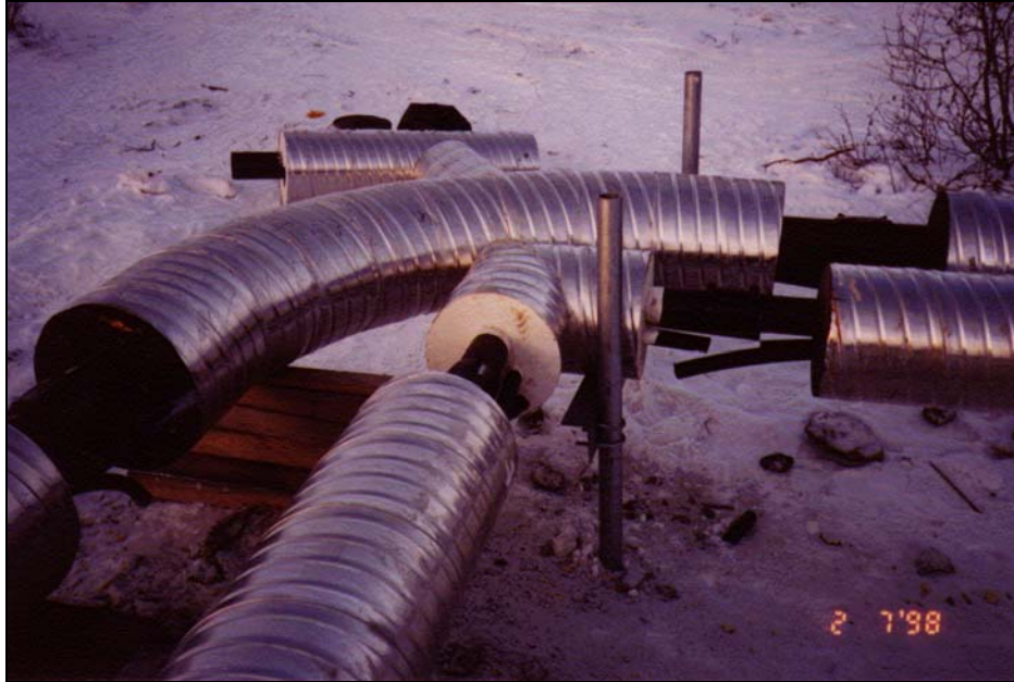
Figure 4.4 Helical Piers in Noorvik, Alaska Installed as Foundations for Arctic Pipe Sewage Installation. The Arctic Pipe Contains a Vacuum Sewage Line. (ANTHC, DEHE)
